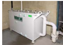
Elevator Sump Pump Interceptors
