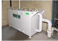
Elevator Sump Pump Interceptors
